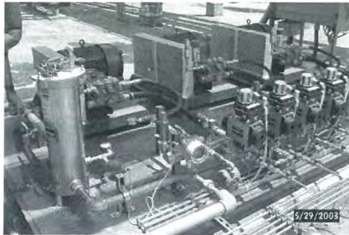
Figure 3 – Wet Compression Pump Skid
