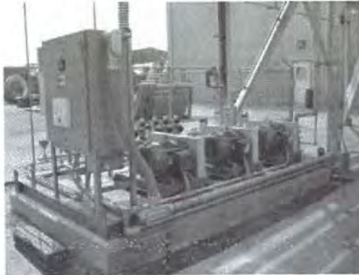
Figure 4 -- Electrical Cabinet with PLC Controller and HMI Interface
