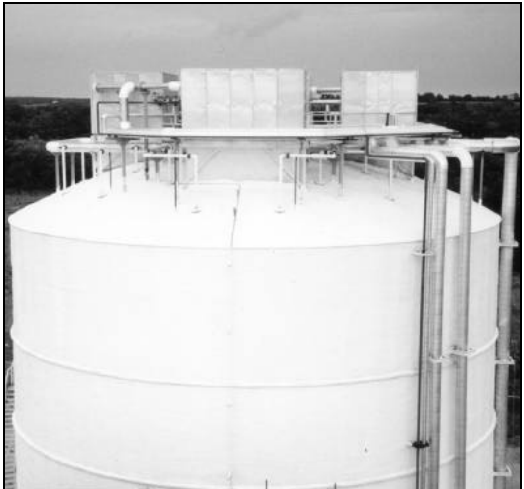
Figure 8: Four enclosed evaporator sections are placed on top of each ice storage.
