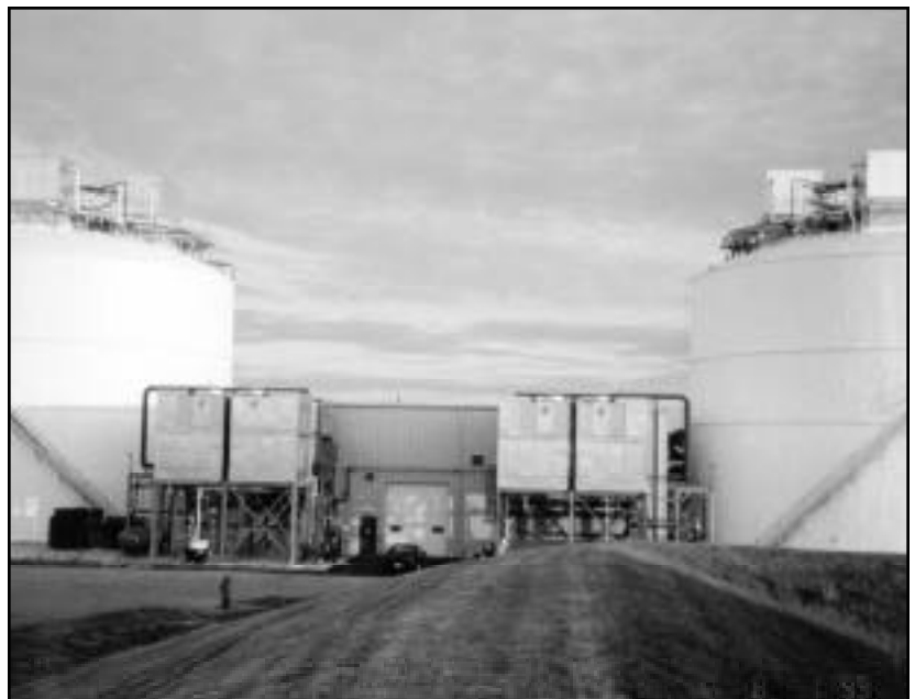
Figure 6: The refrigeration system is placed inside the building between the ice storage tanks.
