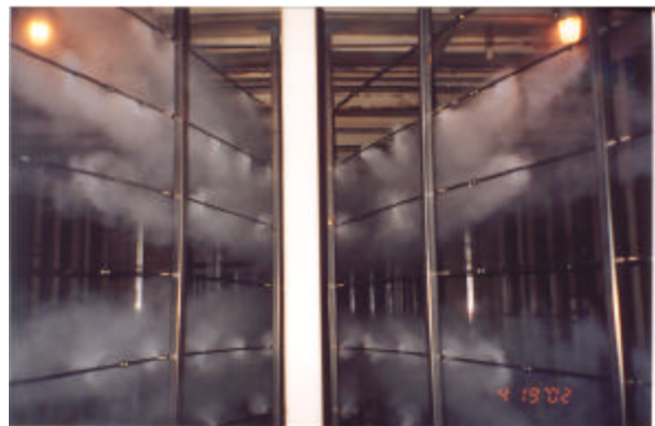
Figure 4: Water spray pattern.
