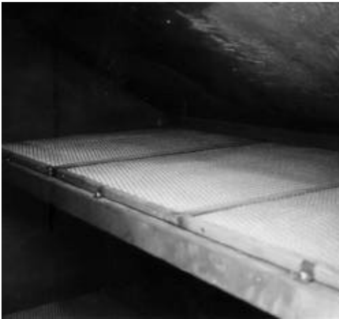
Fig.7: New pre-filters installed to reduce water carryover to final filters.
