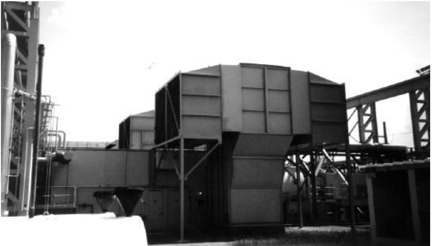
Fig.6: Inlet duct of the combustion turbine after modifications to add weather hoods.
